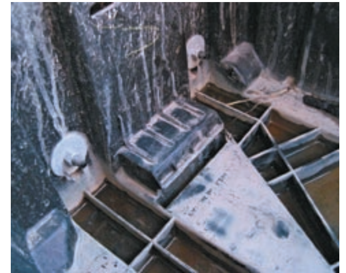
16. Here you see the gussets trimmed flush. This will allow the installation of the new aluminum battery tray.
